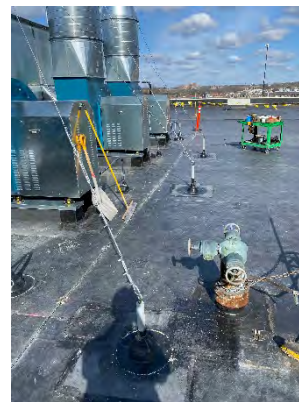
Photo 30: Guy Wire Connections to Roof at Fans
