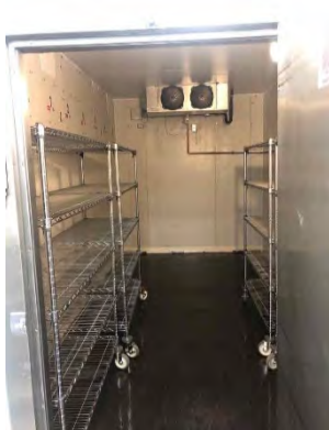
Photo 14: Inpatient Pharmacy – Fan Replaced and Cracks on Floor Sealed with Epoxy Paint
