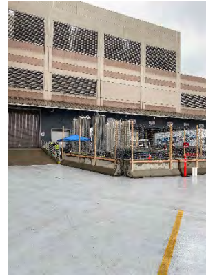
Photo 66: Oxygen Distribution System – Bulk Supply Storage with Jersey Barrier Protection
