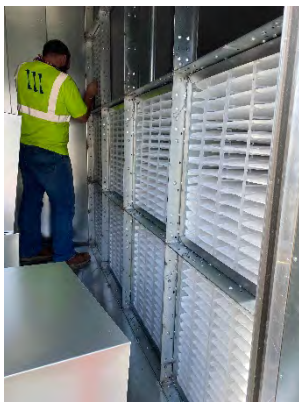
Photo 29: Filters within Exhaust Plenum on Roof
