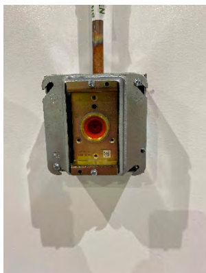
Photo 63: Oxygen Distribution System – Connection at Patient Pod prior to Installation of Cover
