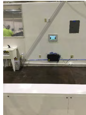
Photo 11: Typical Nurse Station with Handwashing Sink and Associated Supply/Drainage and Electrical and Data System
