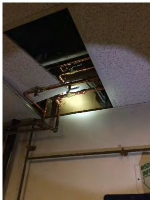
Photo 51: Soiled Utility Room – Soiled Utility Sinks Tied into Existing Domestic Water Above Ceiling Tiles
