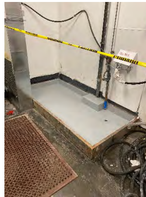
Photo 21: Soiled Utility Room – Slop Sink Sealed to Prevent Leaks onto the Floor
