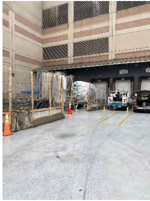
Photo 65: Oxygen Distribution System – Bulk Supply Storage with Jersey Barrier Protection
