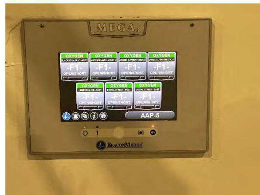
Photo 64: Oxygen Distribution System – Typical Area Alarm Panel
