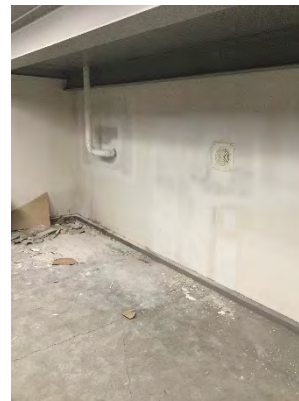
Photo 54: Soiled Utility Room Drainage – Sewage Connected to Existing Sewer through Wall in Emergency Exit Hallway 1 Floor Below
