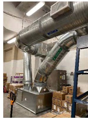
Photo 34: Central Clean Storage – New Air Conditioning Unit to Supply and Exhaust Pharmacy and Clean Loading
