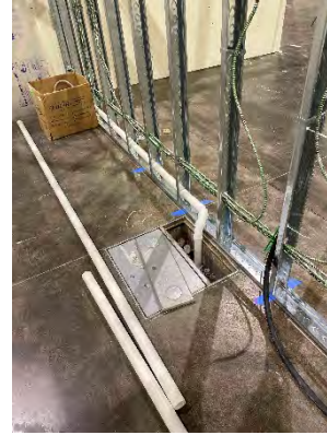
Photo 50: Water Drainage – Connected to Existing Drainage within Floor Boxes in Patient Pods
