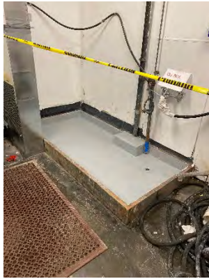
Photo 55: Soiled Utility Room – Existing Slop Sink Resealed to Prevent Leakage onto Floor
