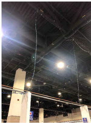
Photo 43: Emergency Power Supply from Catwalk to Nurse Stations
