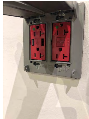
Photo 40: Outlet at Patient Pod – Red Receptacle Does Not Indicate Emergency Power
