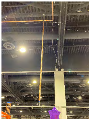
Photo 61: Oxygen Distribution System – Unistrut Column Used to Support Copper Piping at Drop to Patient Pods
