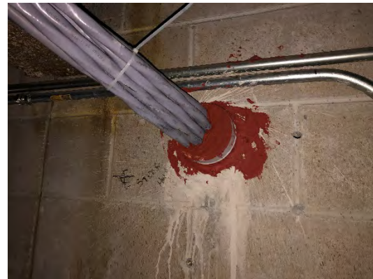
Photo 58: Mechanical Room – Typical Fire Proofing Used at Wall Penetrations for Mechanical Room
