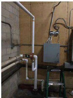
Photo 47: Domestic Water in Mechanical Room – Main Tie-in Point
