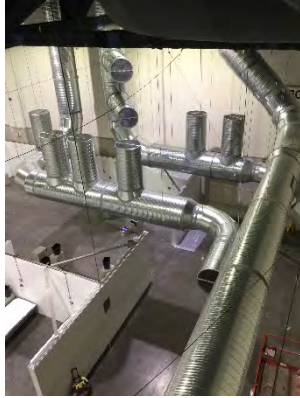
Photo 31: Main Exhaust System below Roof Penetrations
