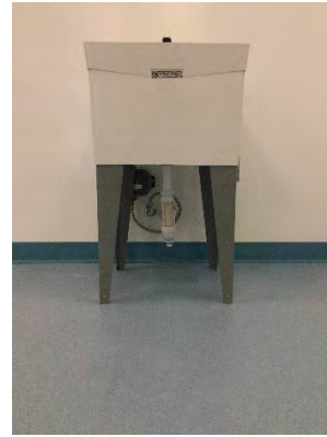
Photo 56: POC Testing Room – New Hand Washing Sink with Supply and Drainage through Wall from Adjacent Bathroom
