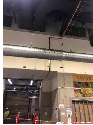
Photo 60: Oxygen Distribution System – Copper Piping Supported at Ceiling Level Until Distributed to Patient Pods
