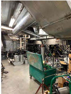
Photo 37: Mechanical Room – Exhaust and Supply for Registration Room Provided by Tying into the Existing System
