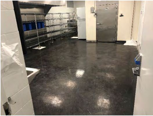
Photo 12: Inpatient Pharmacy – Cracks on Floor Sealed with Epoxy Paint
