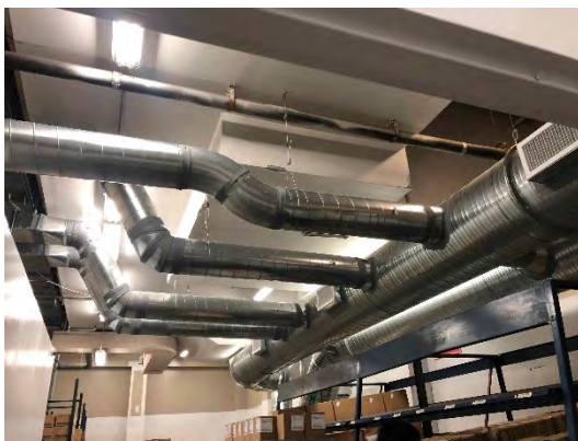
Photo 35: Central Clean Storage – New Supply Ducts for Pharmacy and Storage
