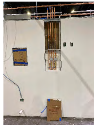
Photo 62: Oxygen Distribution System – Uncovered Valve Box
