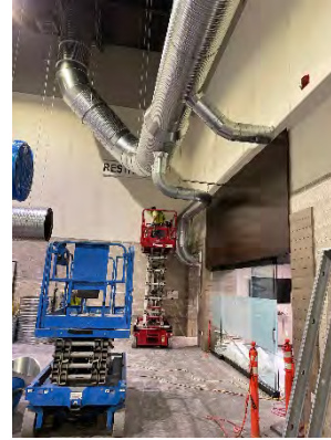
Photo 32: Exhaust Ducts Diverting from Main into Rx Distribution and Northwest Bathrooms
