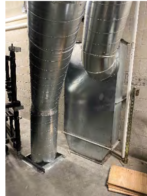
Photo 38: Mechanical Room – Registration Supply Provided through New Floor Penetration and Exhaust Provided by Tying Into Existing Supply Air Duct
