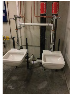
Photo 52: Soiled Utility Room – Two New Sinks Installed and Connected to Existing Water Supply and Drainage
