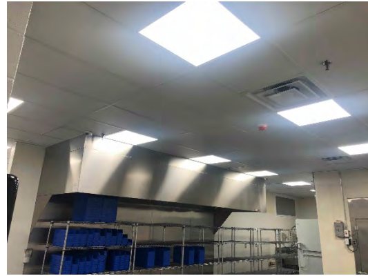
Photo 13: Inpatient Pharmacy – Ceiling Replaced with Gasketed Tiles to Create Air-Tight Room; Security Cameras Added
