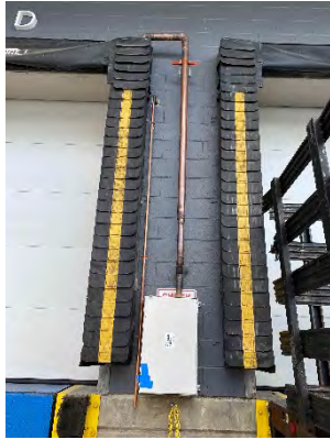
Photo 59: Oxygen Distribution System – Box at Connection to Bulk Supply
