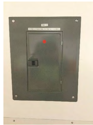
Photo 44: Electrical Panel for Transport Hold Pods Attached to Emergency Power
