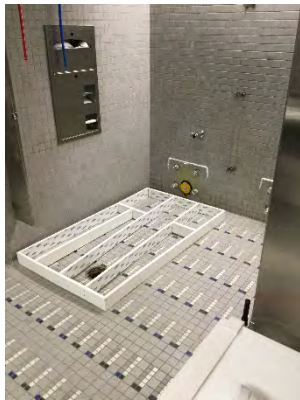
Photo 57: Northwest Women’s Restroom – New Shower Base Constructed to Allow PVC Pipe to Run Directly to Existing Floor Drain
