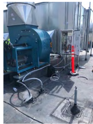
Photo 46: Exhaust Fans – Power Supplied from Emergency System in Mechanical Room; Rooftop Penetrations are Properly Sealed
