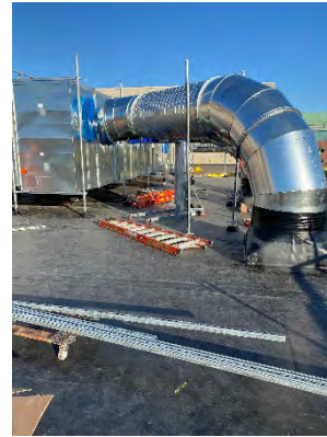
Photo 28: Exhaust Duct from Plenum to Roof Penetration
