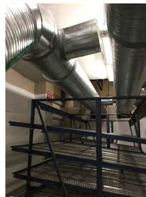
Photo 36: Clean Central Storage – Exhaust Ducts for Clean Central Storage Room
