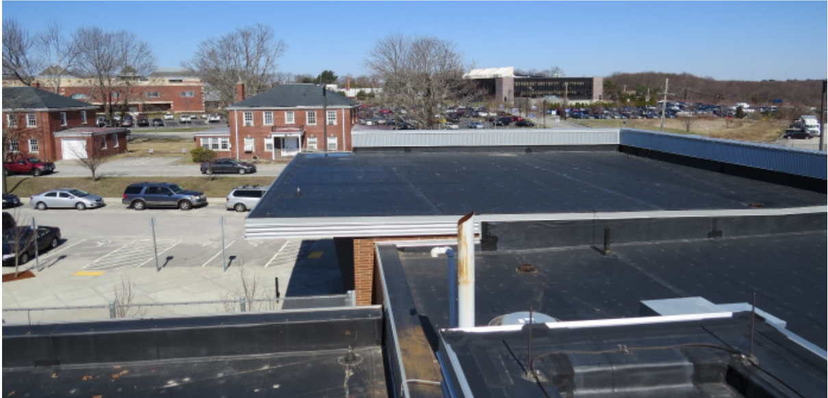
YAC Roof and parapet at Main Entry viewed from the high roof looking west. Area of work scope #23 This photograph is to be referred as detail 5/A102.
