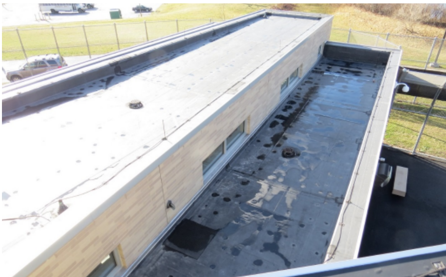
YAC Dayroom A101 Left hand wing, southwest façade, area of work scope #24 This photograph is to be referred as detail 6/A102.
